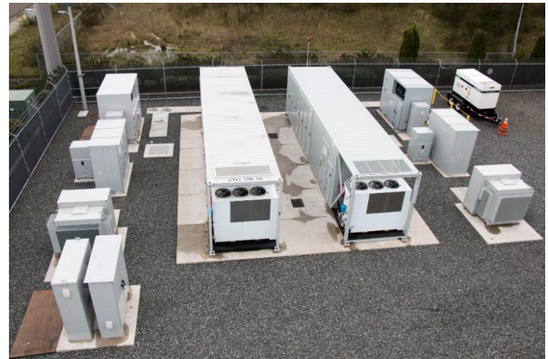
MESA 1 - 2 MW / 1 MWh Li-Ion Battery System in Everett, WA.
