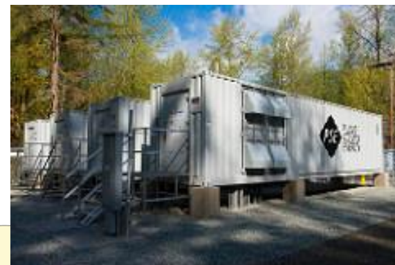
2 MW / 4.4 MWh lithium-ion/phosphate battery – Glacier, WA
