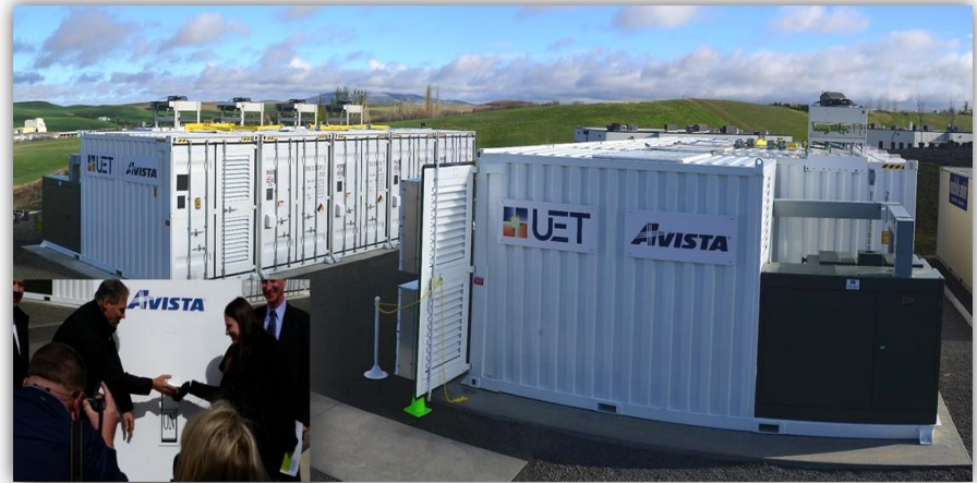
UET Battery System in Pullman, WA
