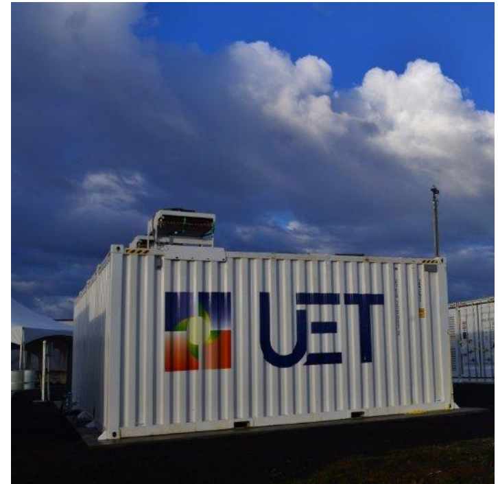
SnoPUD MESA 2 UET 2 MW/8 MWh V/V Flow
