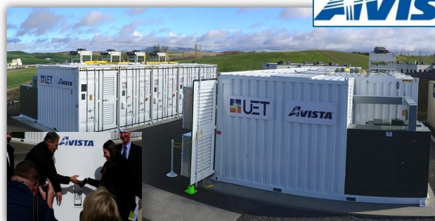
1 MW / 3.2 MWh UET vanadium-flow battery – Pullman, WA
